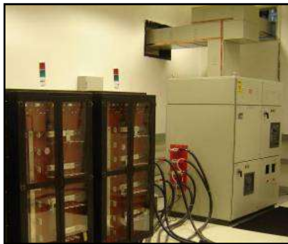
Figure showing Bus bar entry to LT Control Panel and connection to the Make switch and the Load Banks
