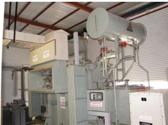
The Short Circuit Testing Transformer
